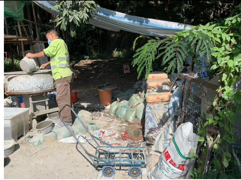
Photo 2 – Dust generating activities (cement mixing) by renovation staff at AM1, Tin Hau Temple. (Taken on 24 Nov 2021)
